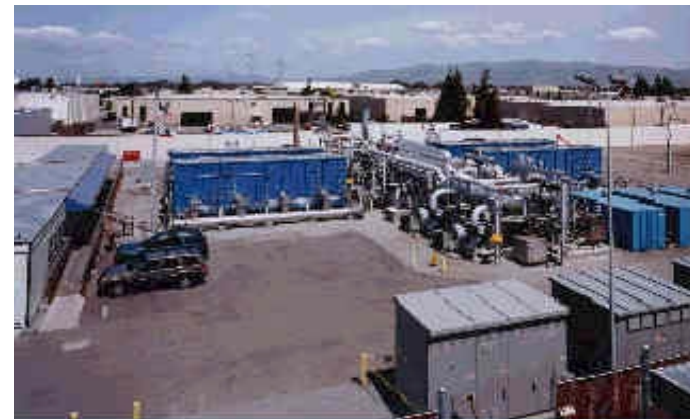
FCE's First Utility-Scale Demonstration in Santa Clara, California, U.S.A.
